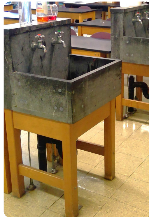
Plumbing fixtures not compliant per ADA (old!)
