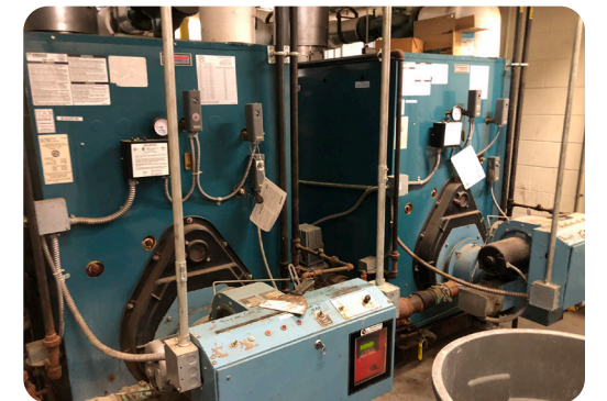
HVAC systems at end of useful service life
