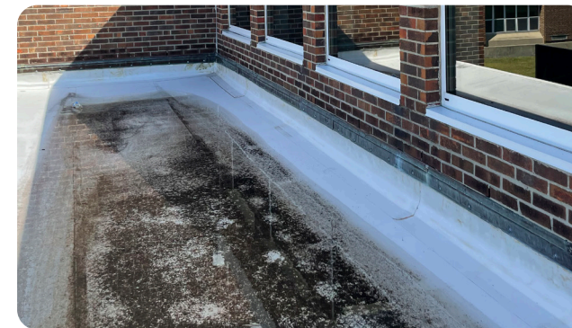
Years of water infiltration at the exterior envelope
